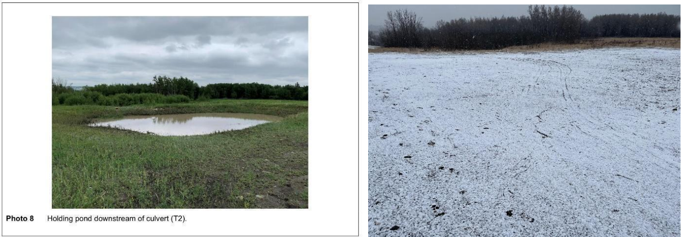
Figure 31. The holding pond after the rain event on July 2, 2021, while the adjacent photo taken on April 19, 2022 shows a large area of un-vegetated mud. Photo 8 from Hemmera’s WAIR.
