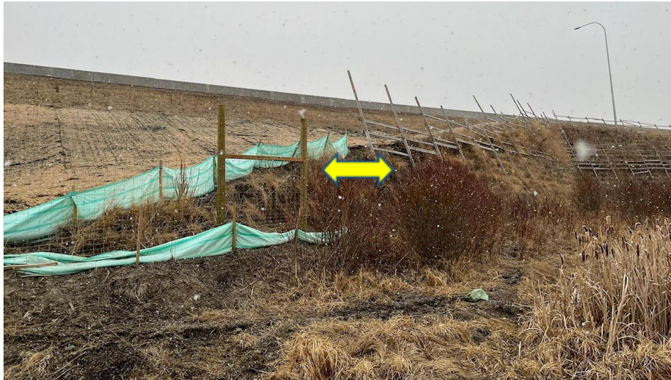
Figure 38. West of the Beaver Pond and south of the retaining wall a visible gap exists highlighted by the yellow arrow.
