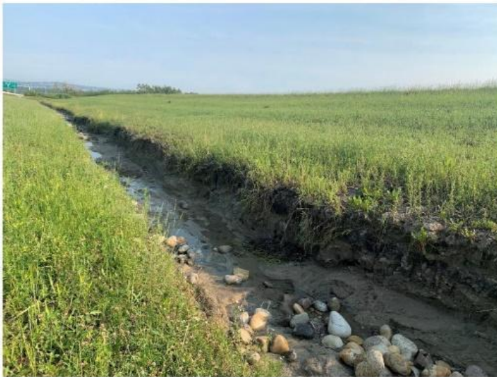
Photo 5 Channel erosion within ditch alignment.
