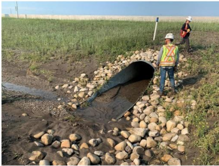
Photo 7 Western culvert berm after rain event.
