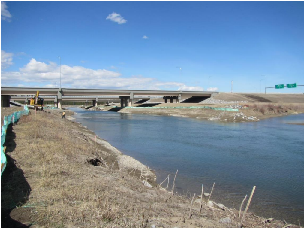
Figure 39. View looking Northwest over the SWCRR showing the wildlife corridors in May 2021 showing construction using heavy equipment along the realignment corridor. Photo taken by Golder during the May 2021 track survey.
